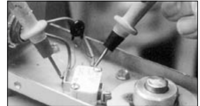
Testing a door switch with an ohmmeter: this type of switch mounts on top of the kiln.
