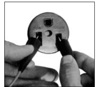
Place voltmeter probes in the two slotted, hot connections of the outlet. The round connection is the safety ground.
