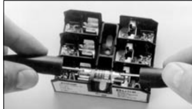
Test a high amperage fuse with an ohmmeter. You can test the fuse without removing it from the fuse holder.
