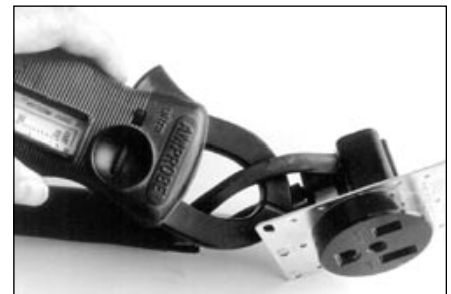
The ammeter attaches to only one hot wire. Be sure breaker is shut off before you remove the receptacle cover.
