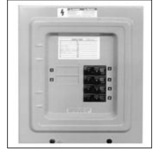
Know the location of the circuit breaker panel. Label the breaker that controls your kiln's circuit.
